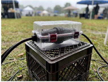
Joint in a cover box, off the ground
